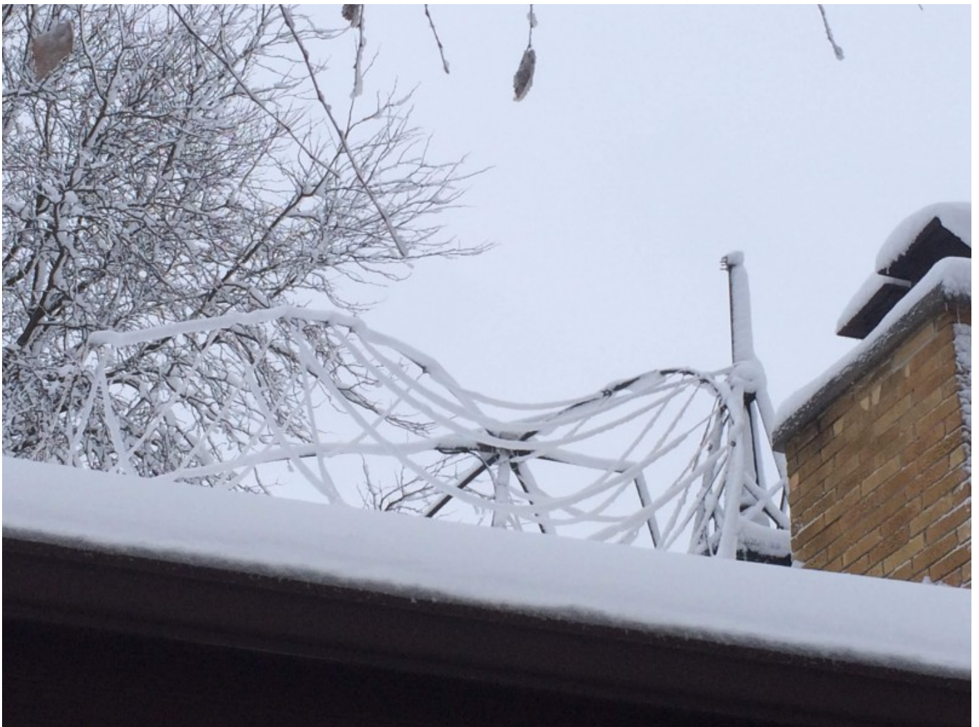
N9JAX had a hex beam come off its mount due to an ice load.
